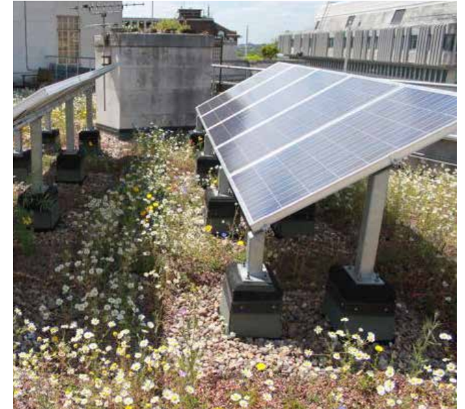
Renewable PV Panels and biodiverse green roof
